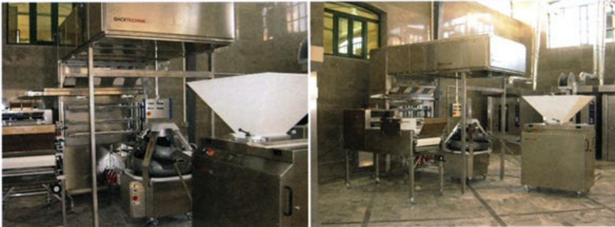
A CPL bread line installation in Iran
